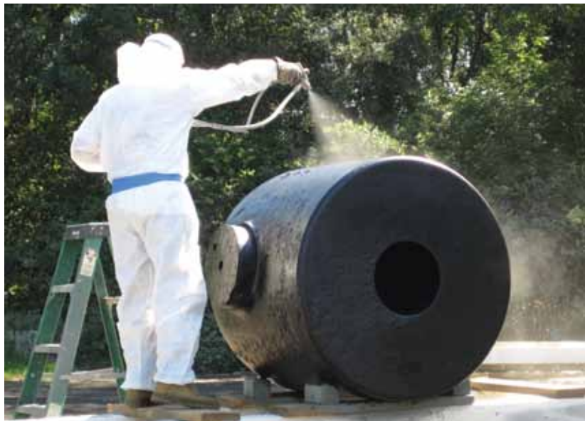
A contractor applies a polyurethane topcoat to a 13-inch seacoast mortar tube.
