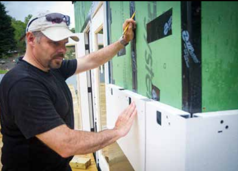
Dan Harding, whose architecture studio formed the project's core, is also an experienced builder. Here, he fits specially designed metal cladding on Indigo Pine East.
