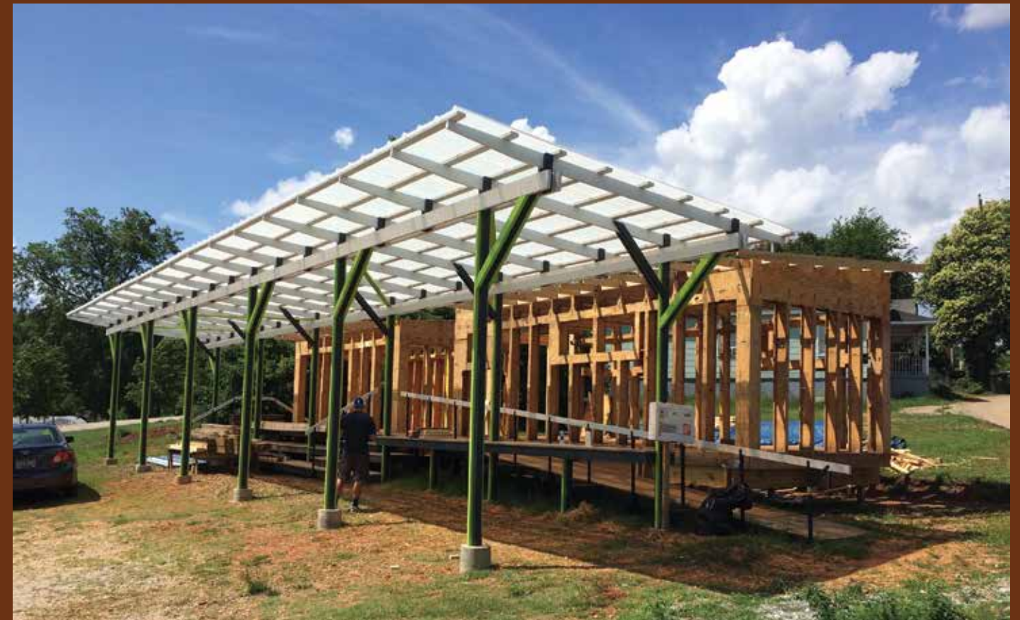
A new Crop Stop, under construction in Greenville, S.C., uses Indigo Pine technology to provide a lot-cost commercial kitchen for local farmers.
